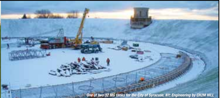
One of two 32 MG tanks for the City of Syracuse, NY; Engineering by CH2M HILL
